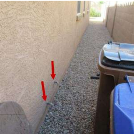
Image 5.4.1 - Discharge pipes on west wall
