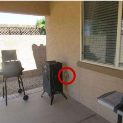
Image 3.9.1 - Broken GFCI Location
