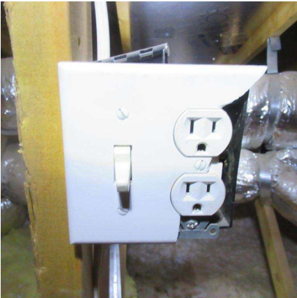
Image 3.11.1 - Broken outlet cover
