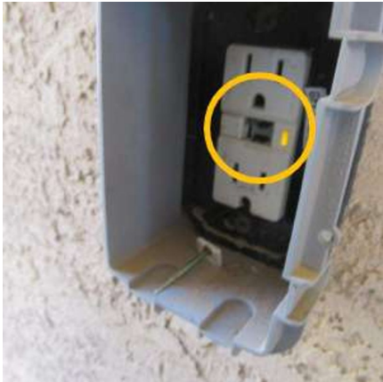
Image 3.9.3 - Broken GFCI Test Button
