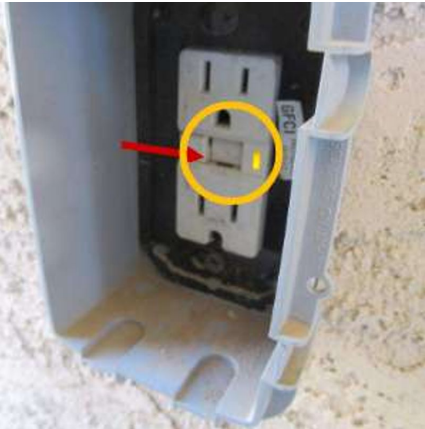
Image 3.9.2 - Broken GFCI Test Button
