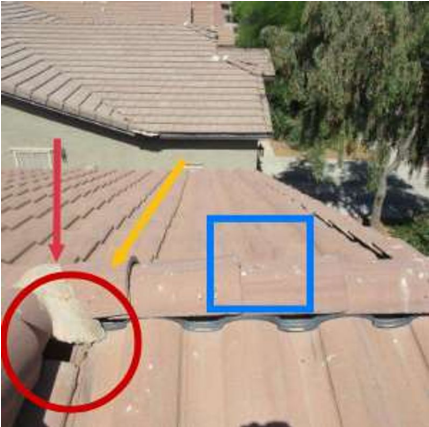
Image 2.2.1 - Roof tile has slid out of place - NE Corner of Hom
