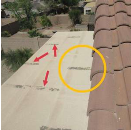
Image 2.2.2 - Peeling coating from joints on patio roof
